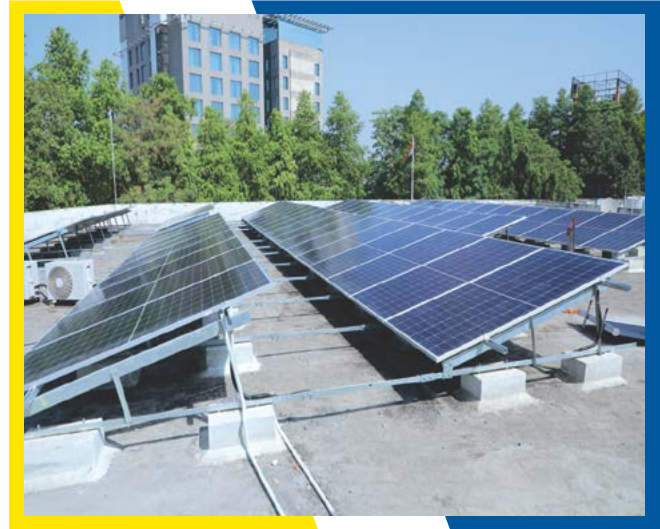
35 kWp capacity Solar Plant installed at Office of Commissioner of Police, Faridabad
