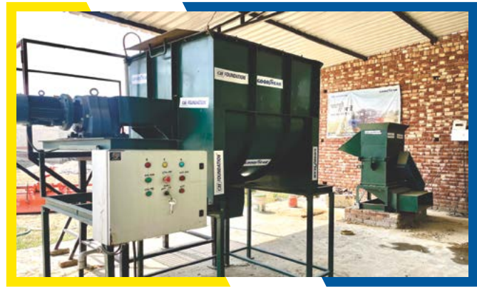
Compost Unit installed at Pandher village, Barnala
