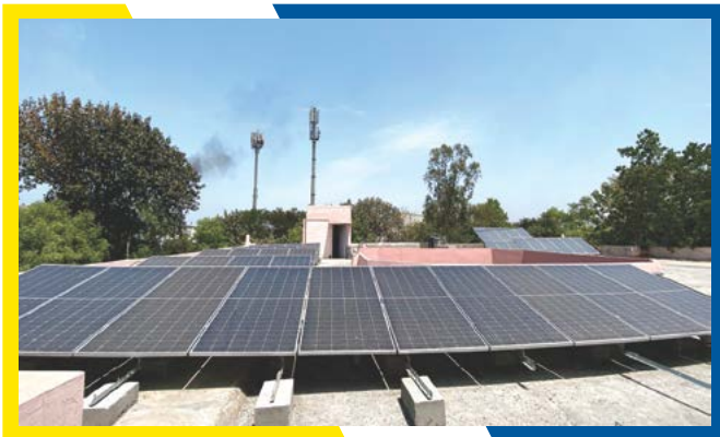
16 kWp capacity Solar Plant installed at Mujesar Police Station, Faridabad
